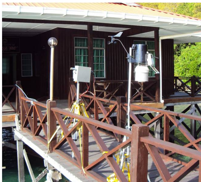
Figure 4.7.: The new telescope unit as installed on Pulau Boheydulang (off the coast of Borneo, Malaysia) performing measurements during SHIVA. In the foreground is a weather station.
